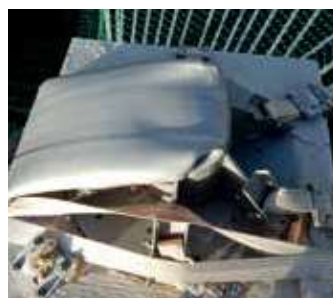
Figure 8: Fixing of the 'additional belts' that have been used for mounting the belt and membranes of the roof structure. Visible are five such belt connections to the stainless steel construction with the sixth one being buried underneath the bent steel structure
