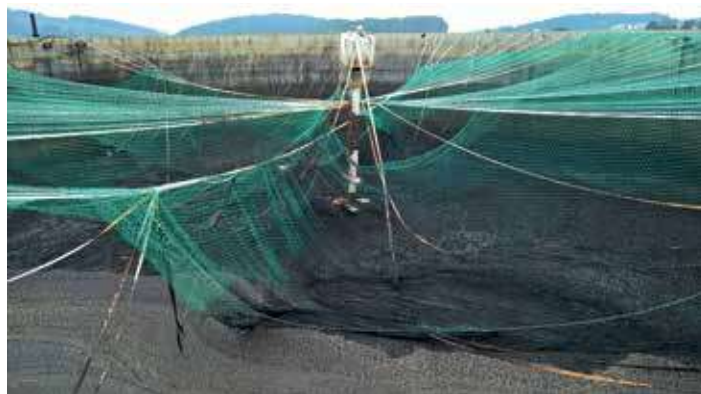
Figure 2: Fully visible centre column, crooked, with massively deformed stainless steel construction on top. Tank still filled with about 1 m of digestate. Net and some belts lying in the digestate
