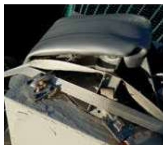
Figure 7: View on the top of the centre column. Massively deformed stainless steel construction. 'Mushroom' bent over to the left. Cracked belt visible on top left of the concrete head of the column
