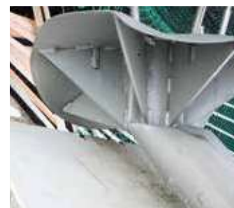
Figure 9: Mushroom head of the stainless steel structure. Bent over the centre column and deformed. On top of the steel structure are visible the sticks that have been used as guidance for the 52 belts laid over the mushroom head
