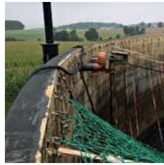
Figure 3: Tank wall with belts still fixed at the wall. Most belts in this area cracked and hanging into the digestate. Left hand side: overpressure/vacuum valve with related outflow pipe (in orange) and mast for submerged mixer next to it
