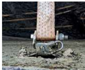
Figure 6: Belt plate, half broken out of the tank wall
