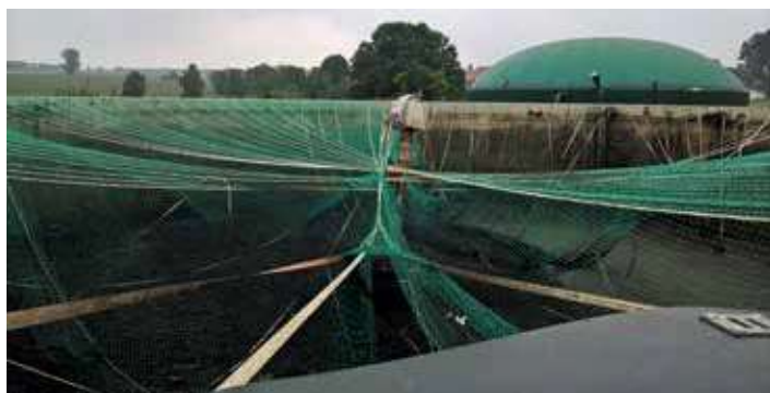
Figure 1: Looking into the digestate storage tank. The gas holder roof membranes already removed. Belts, net, crooked centre column. Background right hand side: secondary digester tank with double membrane gas holder roof
