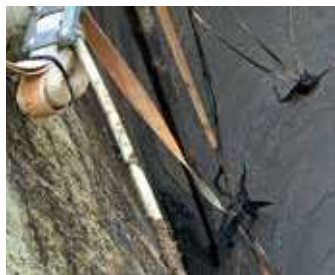
Figure 4: Belts wound around submerged mixer. Top left hand side: belt package with cable tie. For more details details, see Figure 5
