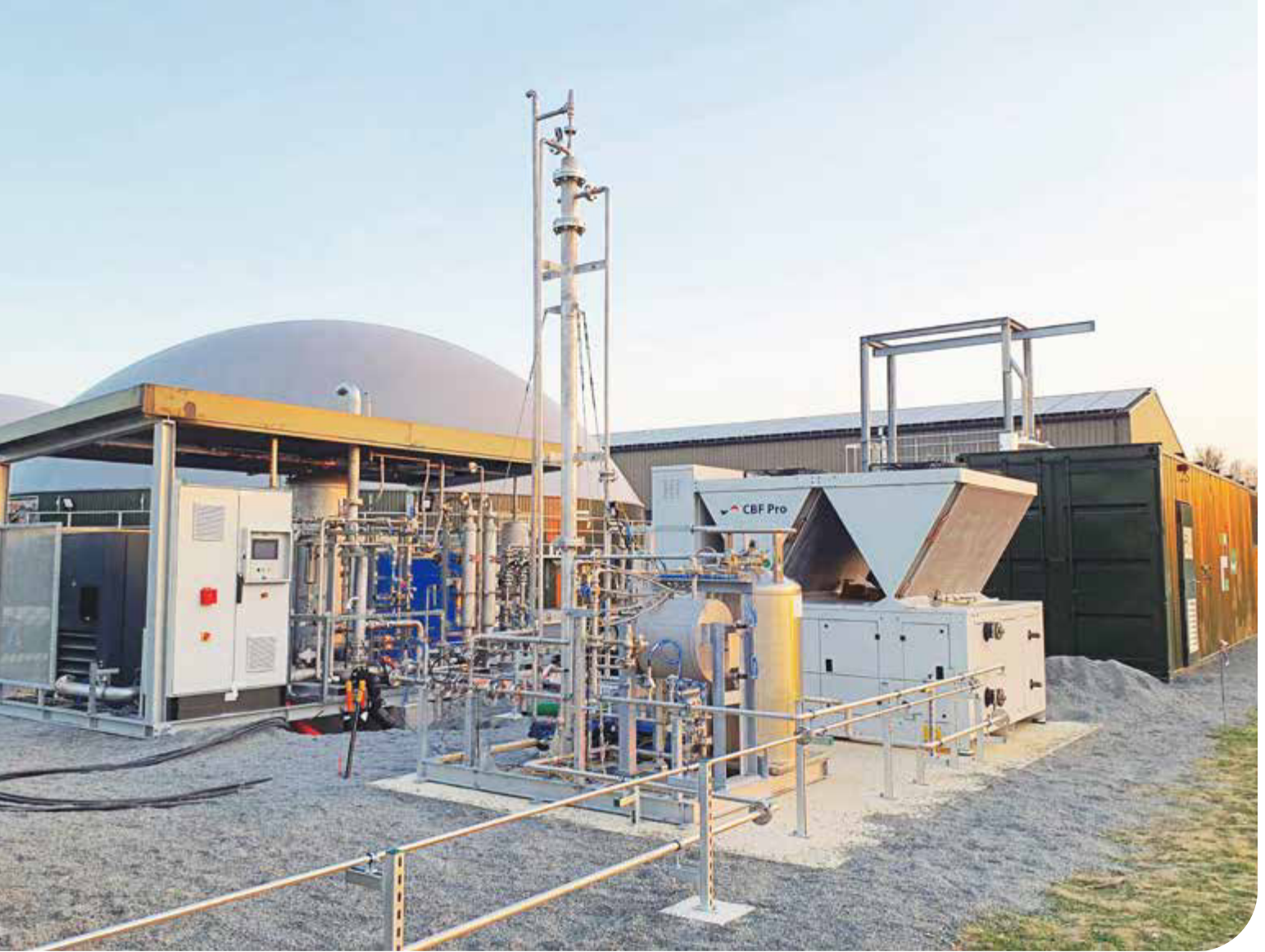
PROVEDAL CO 2 liquefaction system on a biogas plant.
